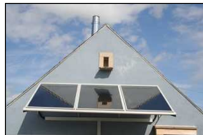
Fig 36. Solar panels at the Battlesteads Hotel, Wark
